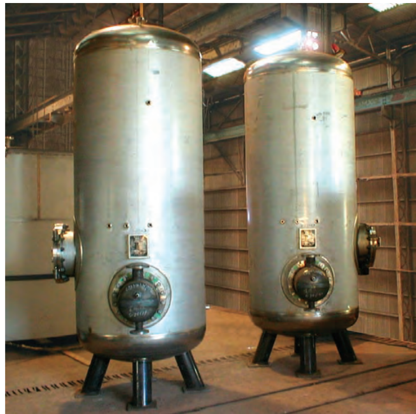
Hot water tanks
